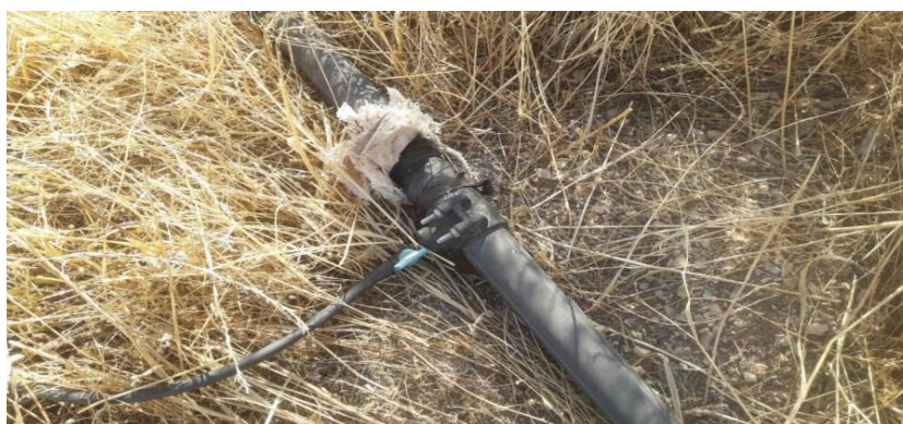
Figure 4. Use of non-standard devices in system equipment
