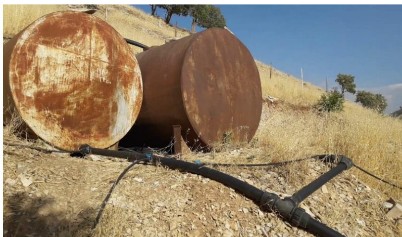
Figure 5. Implementation of the system by people without expertise and use of non-standard devices in the system equipment
