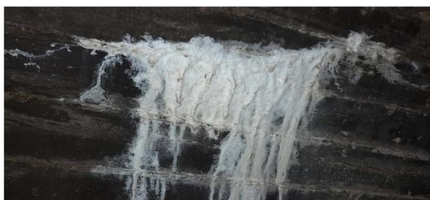
Figure 3. Deposition of Leached materials out of concrete on the wall of spillway's gallery (photo taken in April 2022)
