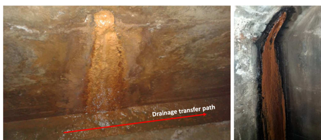
Figure 4. Corrosion signs of embedded reinforcement in concrete structure of Voshmgir dam's spillway (photo taken from operation gallery of spillway in April 2022)
