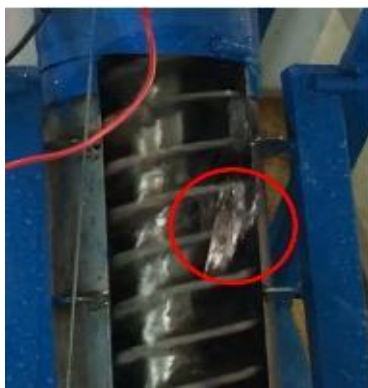
Figure 14. Turbulence by the effects of the welding process
