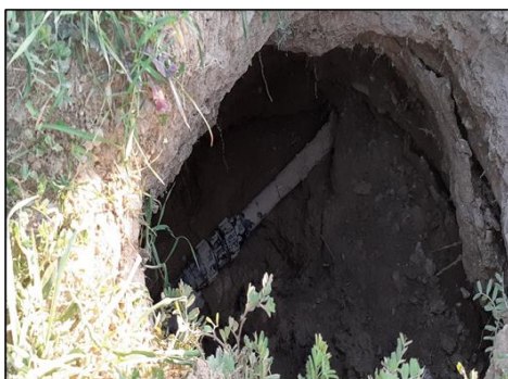
Figure 9. Fracture site in region 6
